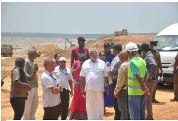
The observation visit made by the Minister of Fisheries on 15.03.2023 in order to provide relief to the fishermen who were employed there due to the complete removal of the water level of the lake to start the development work of the Kalmadukulam lake in Kilinochchi on 15.03.2023
