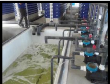
water recirculation system
